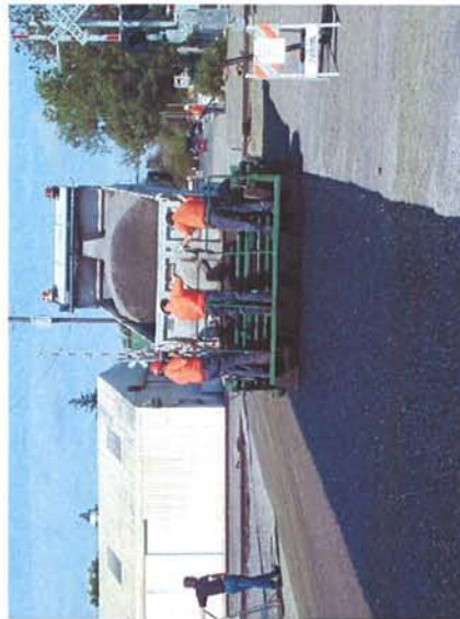
The rock is applied from a spreader box attached to a dump truck driving in reverse.
