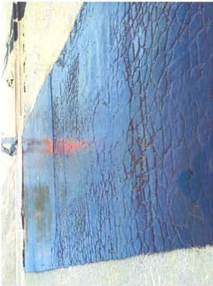
Initial application with the oil truck. PASS® emulsion penetrates the severely cracked surface of the old roadway. Very little preparatory work preceded the application.
