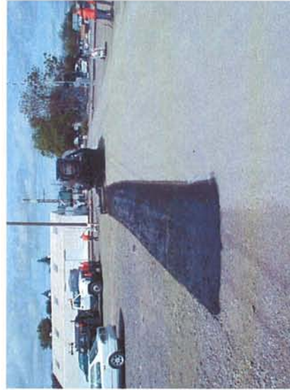
To widen the road and prevent some dust the double chip seal was applied over native soil and rock adjacent to the roadway.
