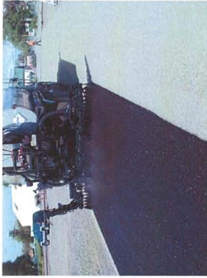
Spray truck applying the second layer of PASS® emulsion over the first layer of rock.
